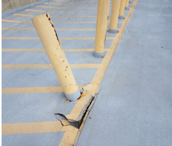
Figure 5 - Common Concrete Damage
