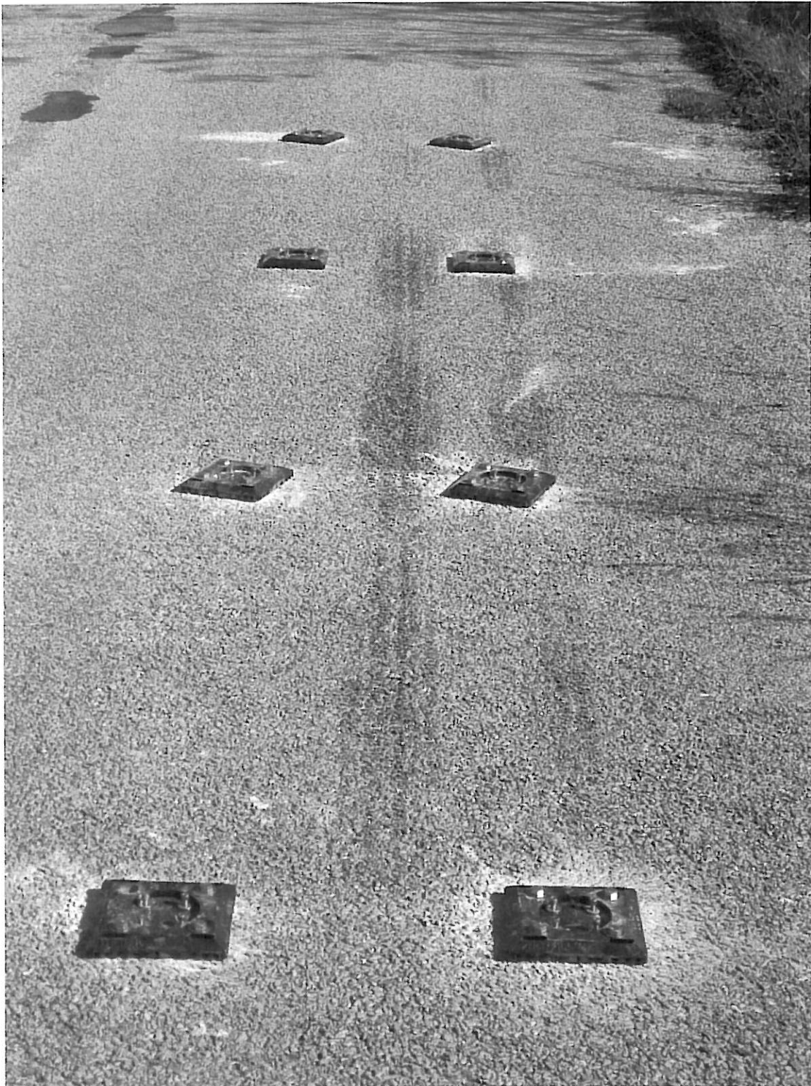
Photo #1 #101 Fixed Bases, installed, depicting the second and fourth row of bases installed at a 25 degree slant.
