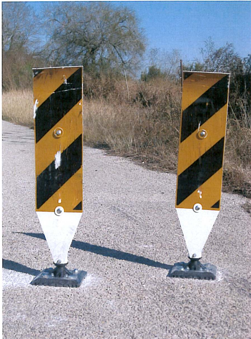
Photo #12 10 impacts completed. 8 Object Markers remaining. 95% of sheeting remains intact. No listing.
