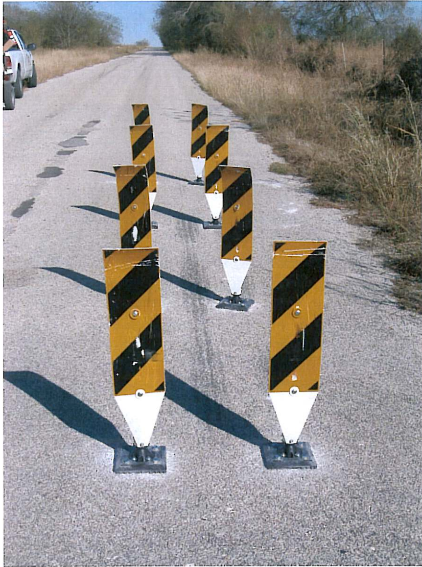
Photo #6 5 impacts completed. 8 Object Markers remaining. 95% of sheeting remains intact. No listing.
